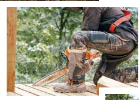
Once all the underfoot bars have been laid, the edge is "Smoothed out" using the saw.
